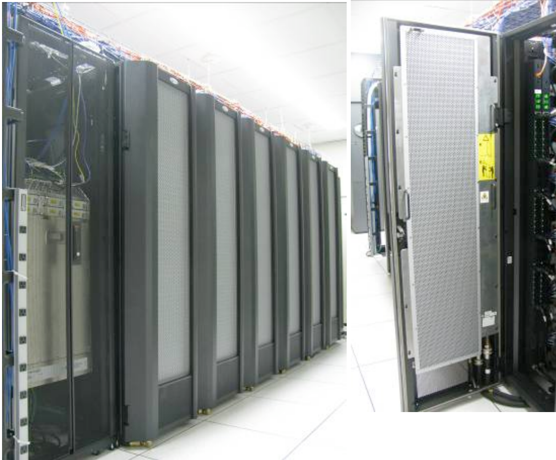
Dedicated Chip cooling loop →
